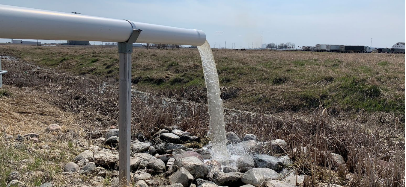
Figure 1. The NDSU Langdon Research Extension Center Groundwater Management Research Project Lift Station.
