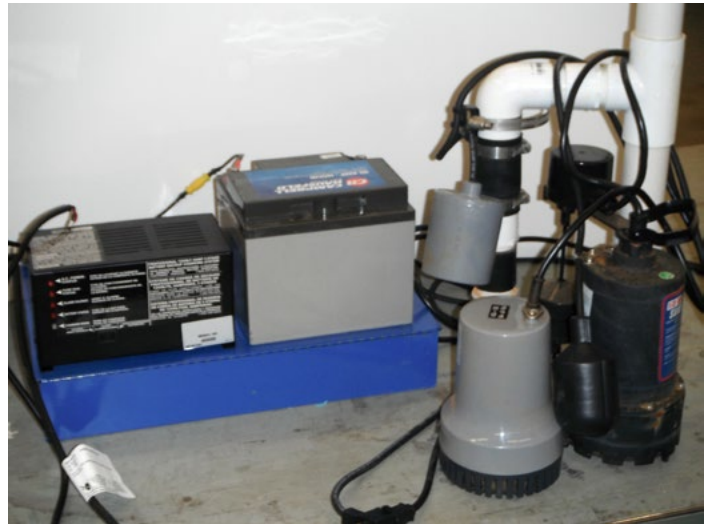
Figure 7. Charger and battery with the primary and backup pumps.
