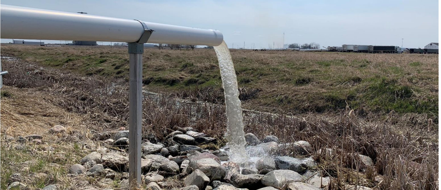
Figure 1. The NDSU Langdon Research Extension Center Groundwater Management Research Project Lift Station.
