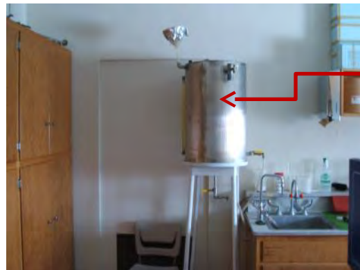
Temporary water storage
