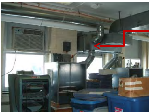
Inadequate, temporary ventilation added to research lab
