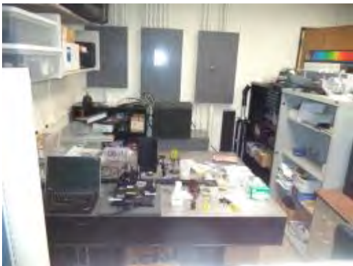
Electrical room converted to faculty/research lab
