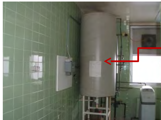
Water treatment equipment in men's restroom
